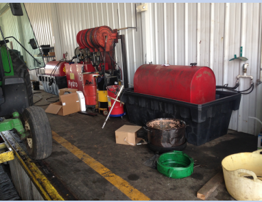
Figure 11: Clifton Facility petroleum storage indoors with secondary containment
