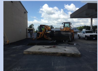
Figure 7: Vehicle wash bay separator cleaning
