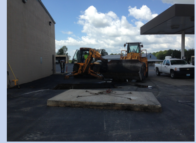
Figure 7: Vehicle wash bay separator cleaning
