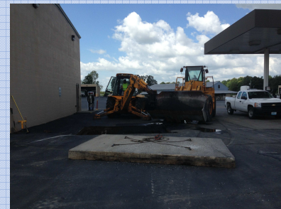
Figure 24: Vehicle wash bay separator cleaning
