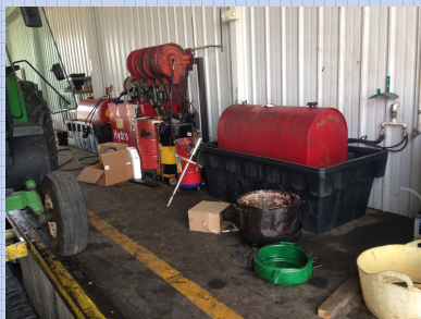
Figure 27: Clifton Facility Petroleum storage indoors with secondary containment
